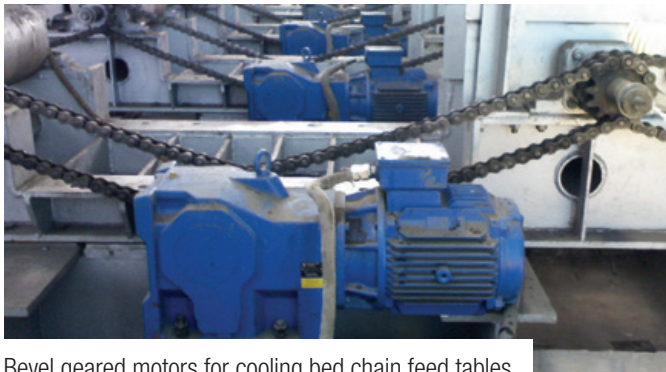
Bevel geared motors for cooling bed chain feed tables
