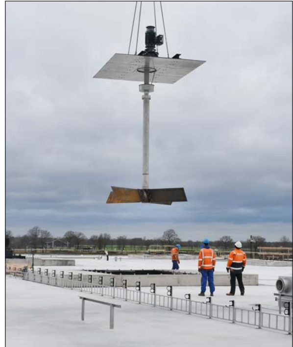
Right: The agitators are lifted to the roof of the fermentation plant by a crane.
